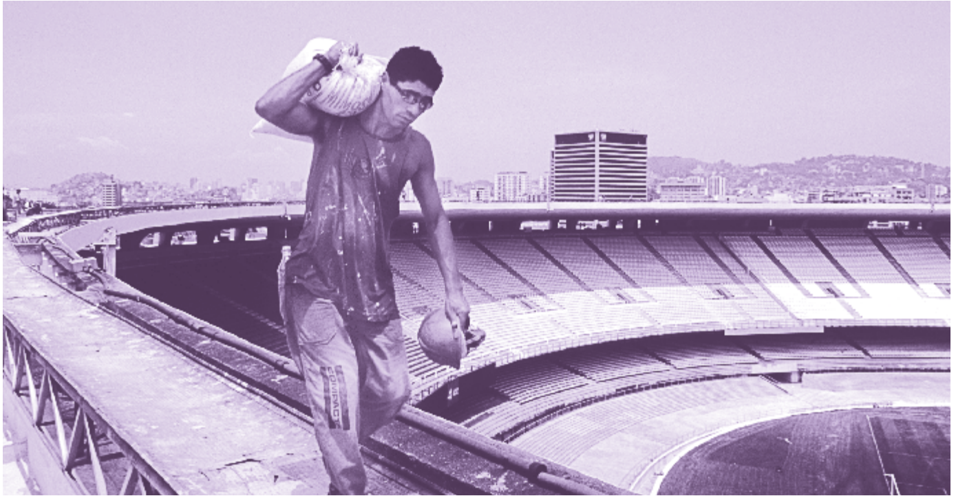
FIFA demanded that twelve stadiums be renovated or constructed for the World Cup in Brazil: the Maracanã stadium in Rio during renewed renovation works in 2013.
